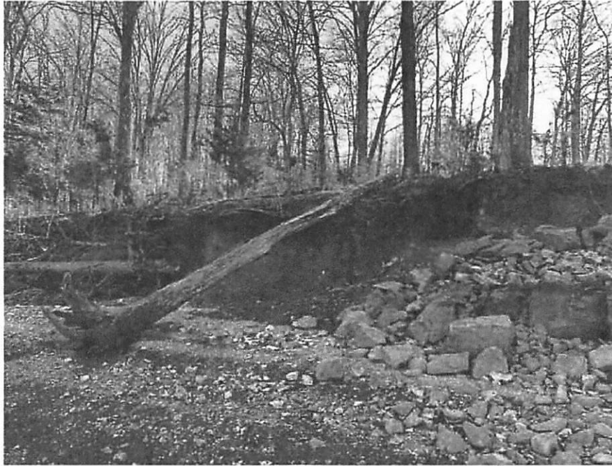
Photo 13: Eroding banks along armoring area 2
